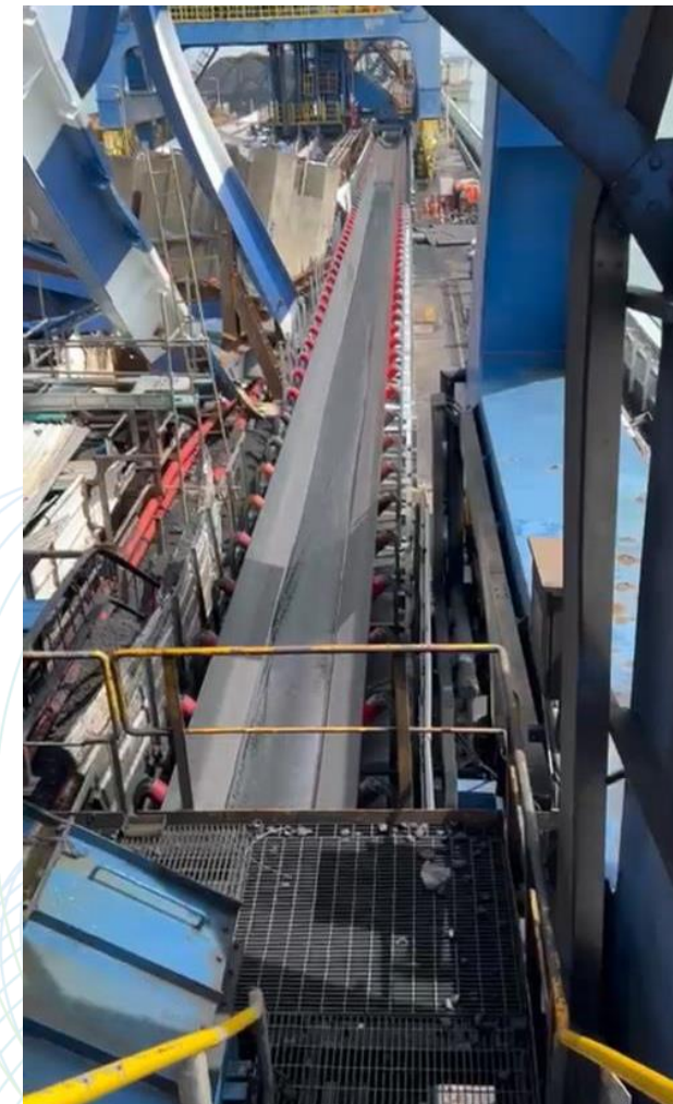
Conveyor belt line C in operation
